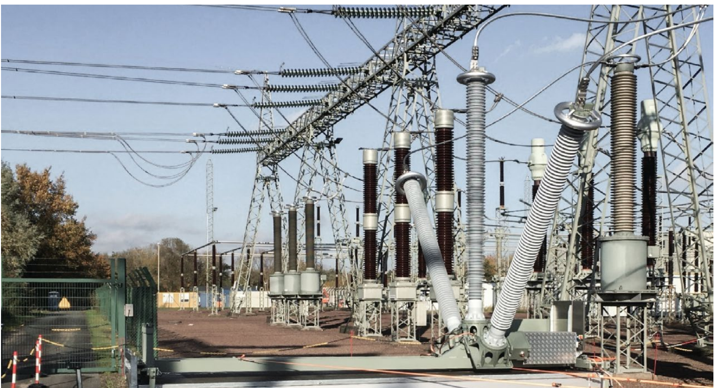
Figure 5: Mobile RC-divider for temporary measurement of power quality in the transmission grid (substation Unterweser)
